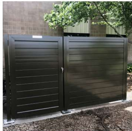
METAL GATE FOR THE MECHANICAL YARD
