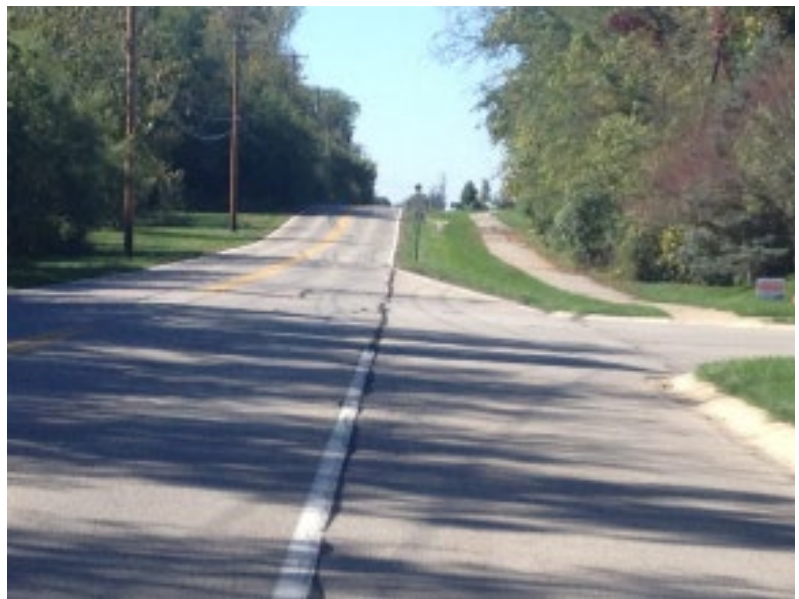
121st Street is an example of a Collector Road with a path only on one side.
